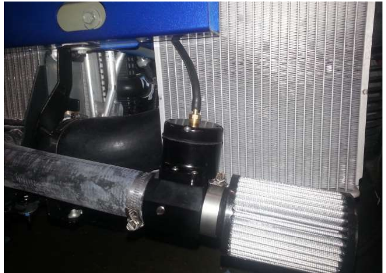
Vacuum Line Connected at Surge Valve
