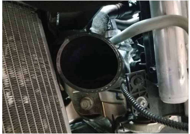
Blower Discharge Tube Installed
