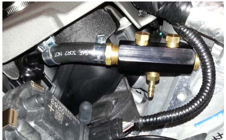
Vacuum Manifold Top Port Installed
